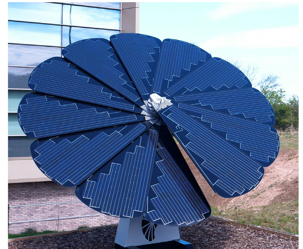
Fig. 24 - Existing solar panels installed on SEZ site.
